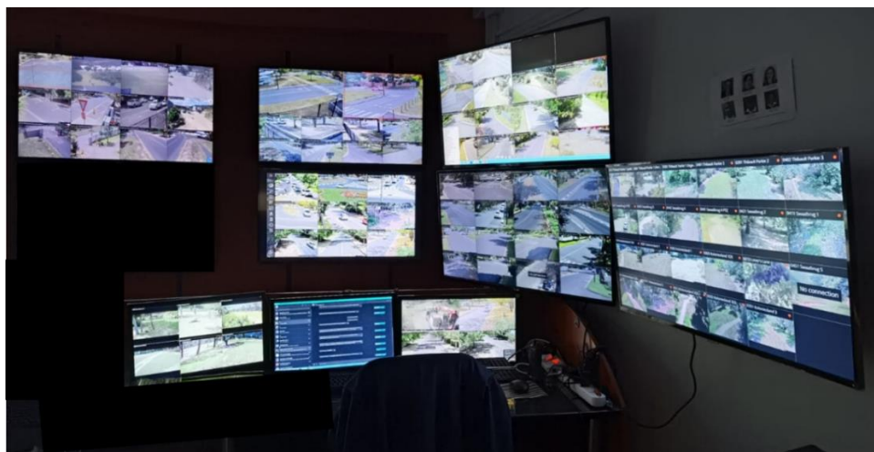
View of the monitoring screens in the JSRA Control Room
